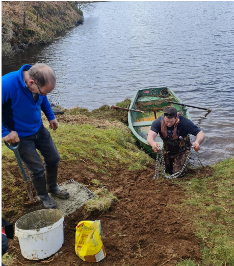
Allan concreting the top of the gabion, while Andy sorts out the chain loop.
